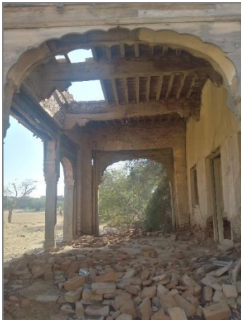
Figure 21: Multi-foiled arches at the fort has been damaged (Source: Author)
