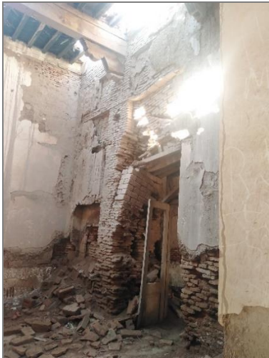
Figure 24: Roof and walls of the room have damaged (Source: Author)
