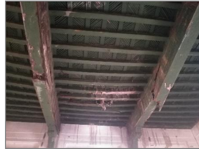
Figure 17: Hardwood ceilings of rooms has been destroyed (Source: Author)
